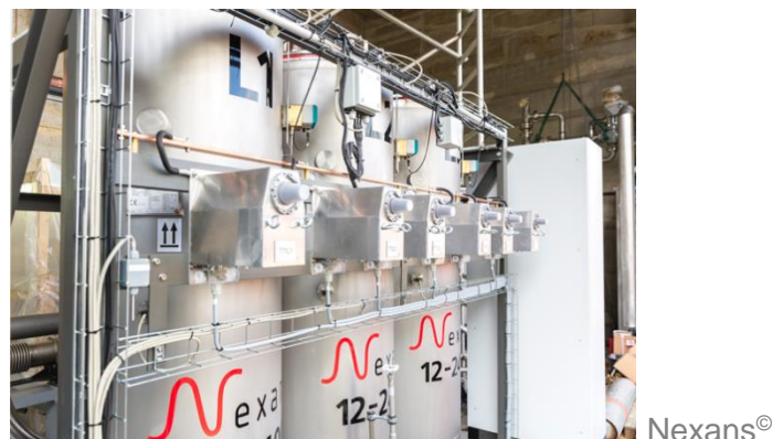
Figure 1: Nexans SFCL in a 10 kV substation of Essen (Germany) in operation since 2014.
